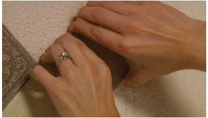
To remove a tile, pull it back and down from the wall.
